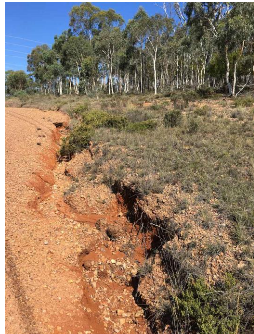
Fig. 12. This 50-cm deep channel along the edge of the Powerline Track has been caused by exposure of the erodible red clay B horizon. Photo: R Purdie.
