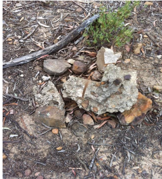
Concrete from the "no-cycling" sign post, showing mark where one of the bolts had been
