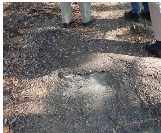
Photo Jean Geue Summit walk surface needs replacement
