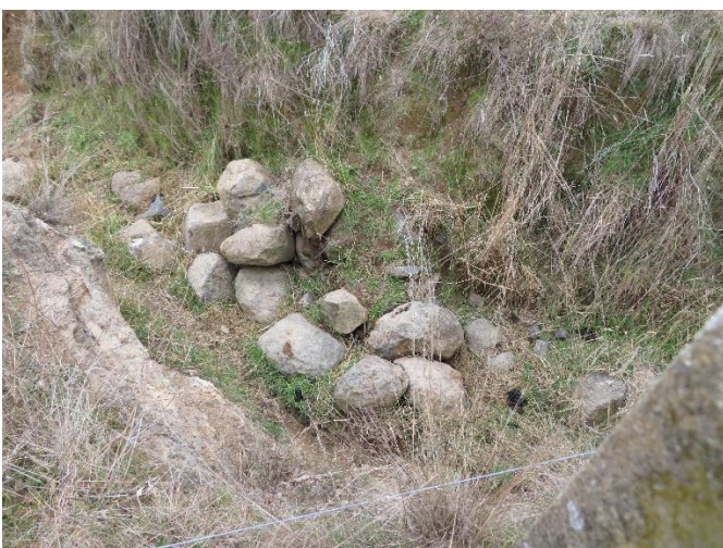
Rocks waiting to be used for construction of convex structure by PCS
